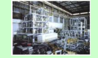
Helium Engineering Demonstration Loop (HENDEL)
