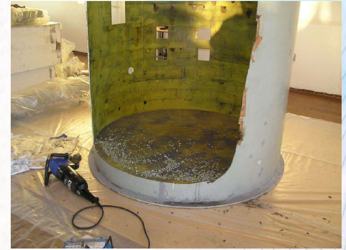
The nibbler and the half-cut reflector tank
