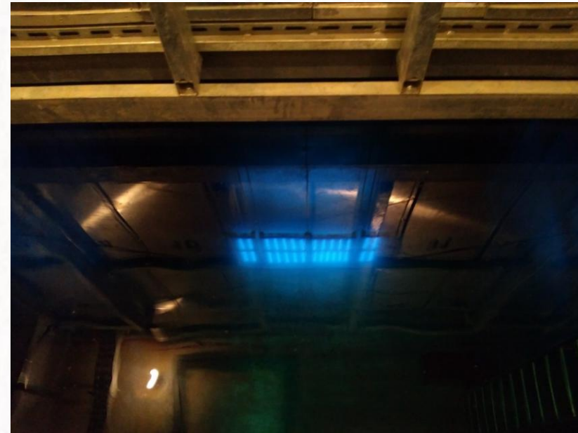
Source Rack / Rak Sumber
