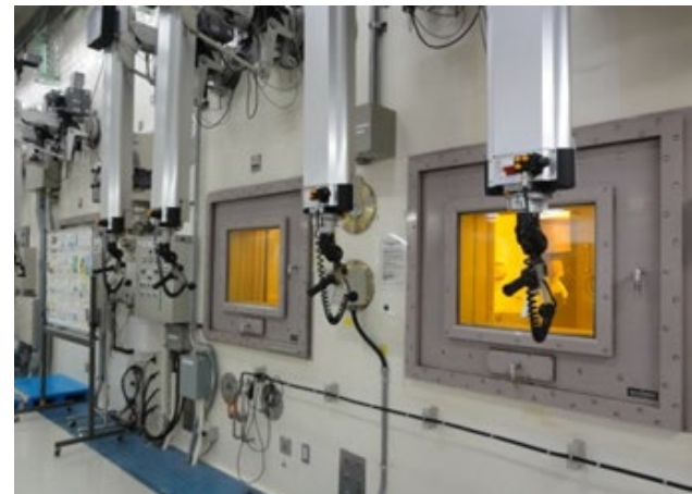
Concrete cells for high level radioactivity
