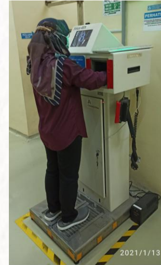
Hand and Foot Monitor Monitor kontaminasi tubuh
