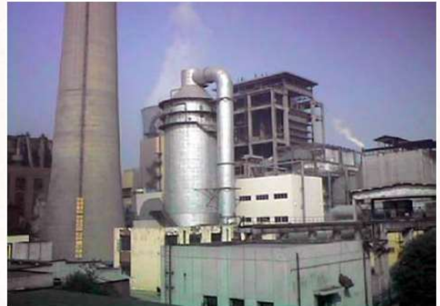
Flue gas cleaning plant in Chengdu, China.
