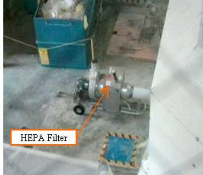
Figure 24. HEPA Filter Set-up
