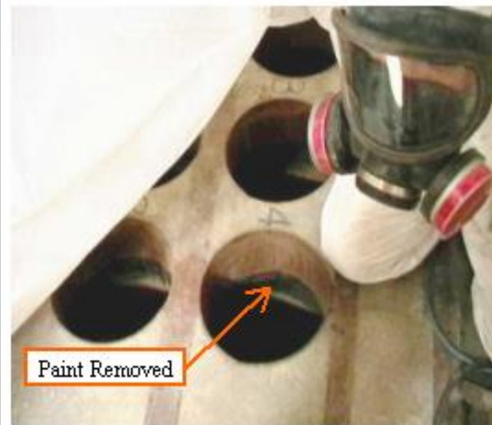
Figure 27. Fuel Storage Pit
