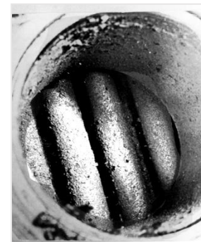
Slag deposits in The Heat Exchanger
