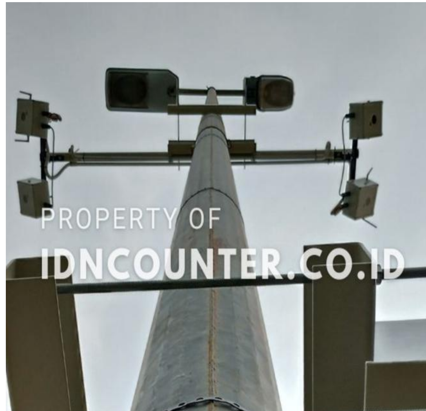
Traffic Counting System Murata Manufacturing, PT. Agrisinar, BRIN
